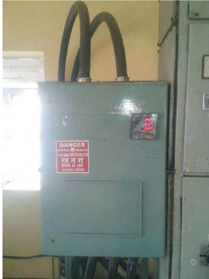
Electric energy meter for E.T.P.
