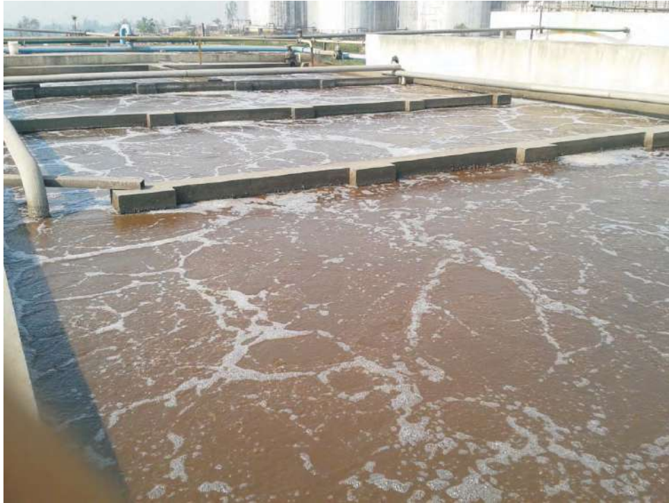
Old diffuse aeration tank
