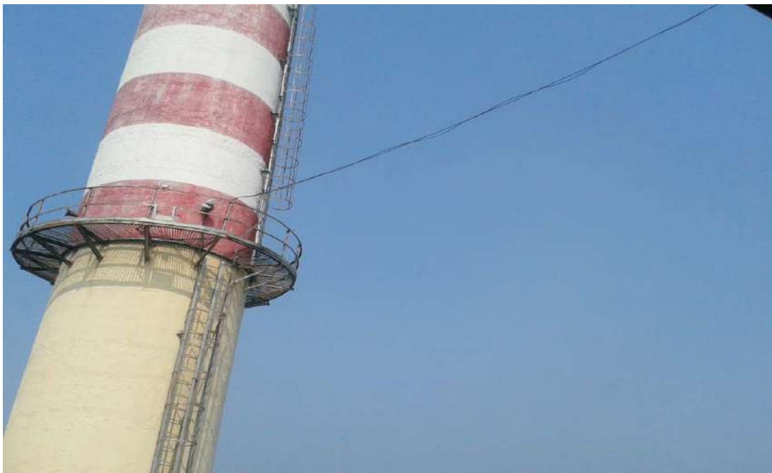
Dust monitor unit for Total Particulate Matter for 72 mtr.height stack
