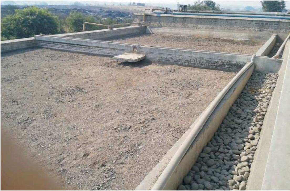
Sludge Drying Bed
