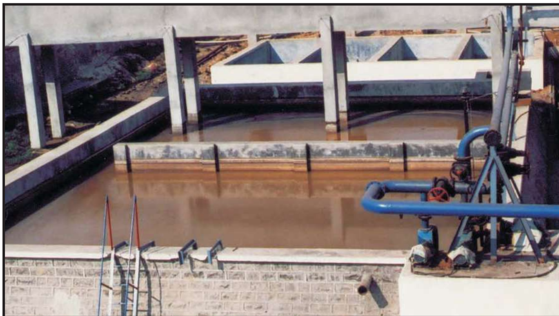
New equalization tank and feeding system to old and new stream 20 M 3 /hr.+ 70 M 3 /hr.
