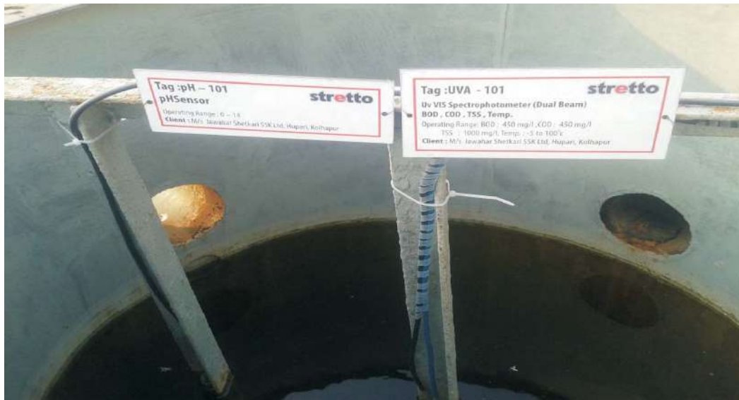
Sensor for outlet Treated Water -for parameter pH, T.S.S, C.O.D & BOD measurement.
