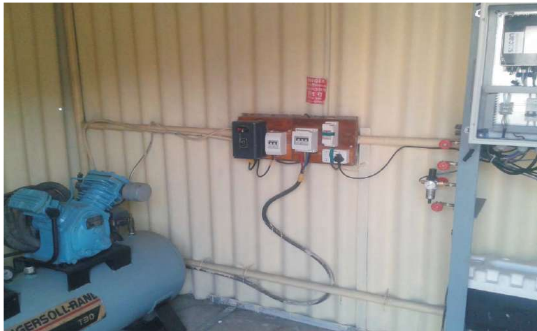
System for Treated Water Monitoring
