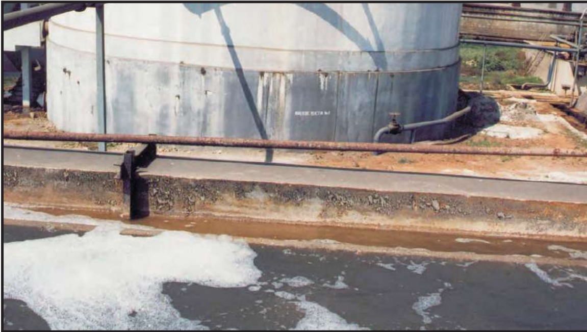
New anaerobic counter current digester 70 M 3 /hr. and preareation tank outlet
