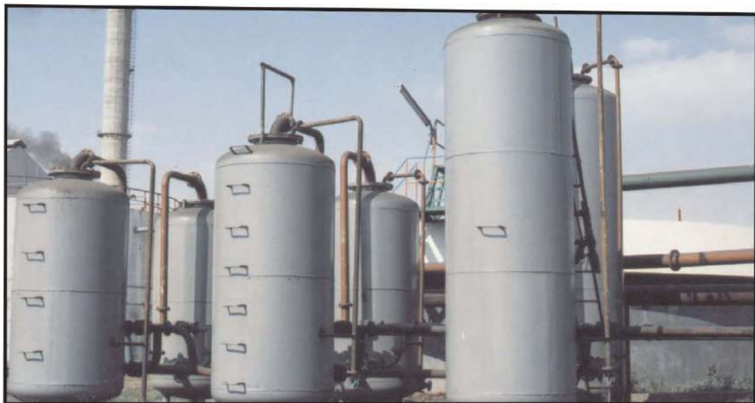
Tertiary system to streams 100 M 3 /hr. each Power sand filter followed by plant based activated carbon & polishing unit comprising high grade anthracite and activated carbon
