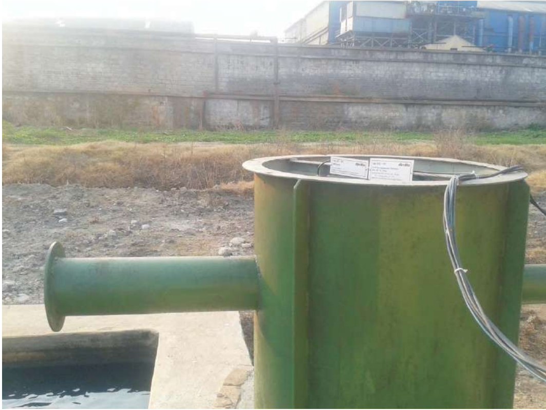
Treated Water outlet Tank
