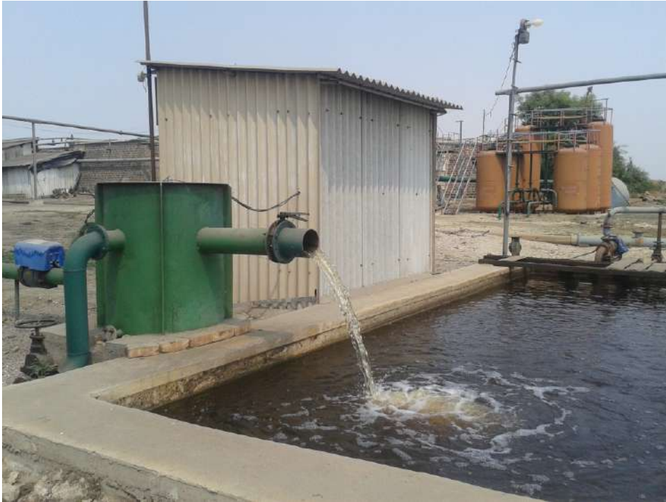
Treated Water Outlet
