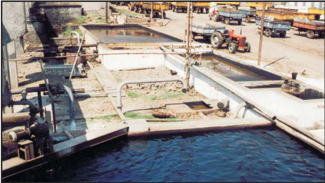
Two stage primary to remove oil & sludge and old equalization tank
