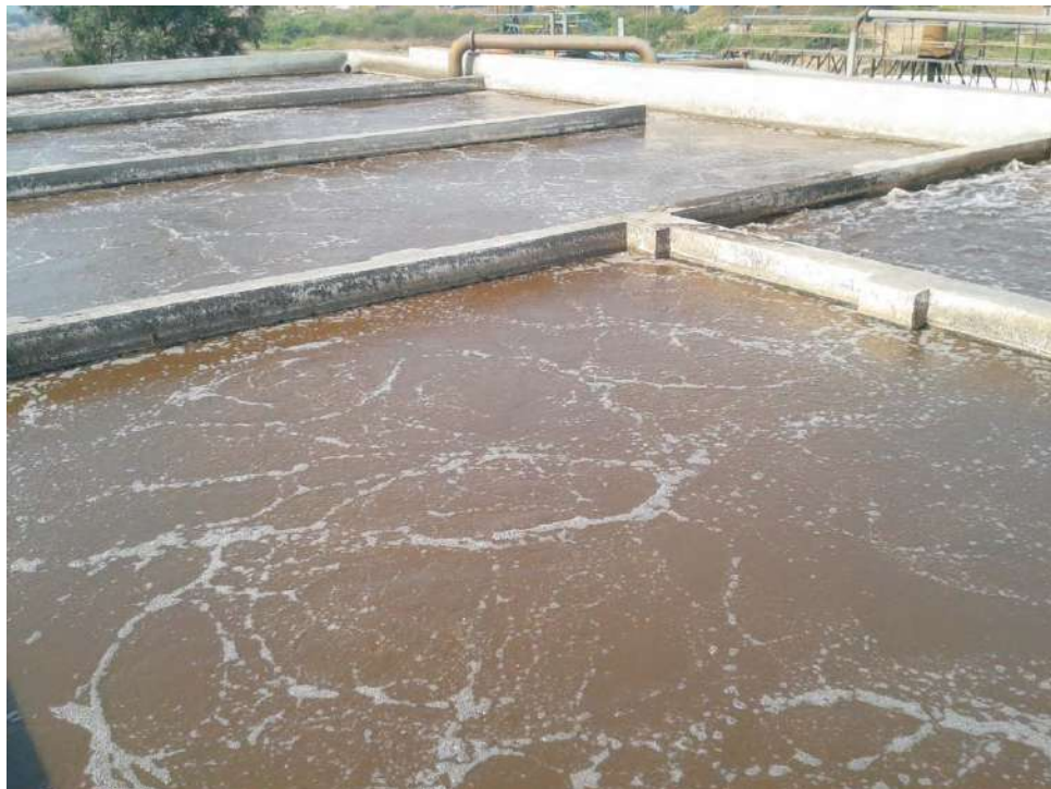
New diffuse aeration tank
