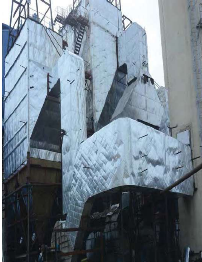
Electro Static Precipitator for 20 M.T/hr Boiler Capacity
