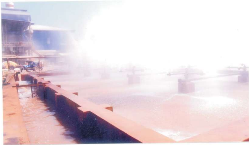
Mini spray pond capacity 10200 M 3 /day water recycle inlet temperature 58°C to 60°C outlet temperature 28 to 30°C
