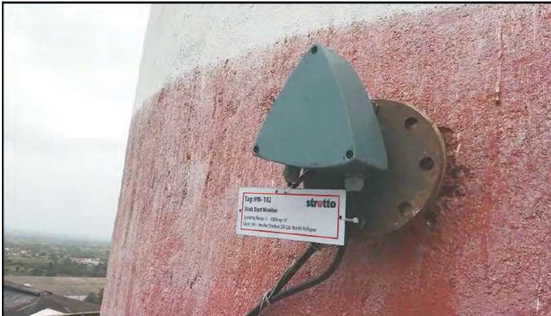
Dust monitor unit for Total Particulate Matter for stack
