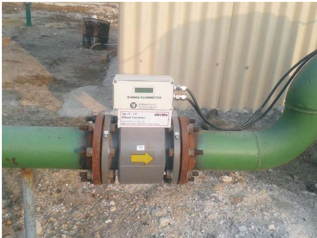
Flow meter for outlet Treated Water
