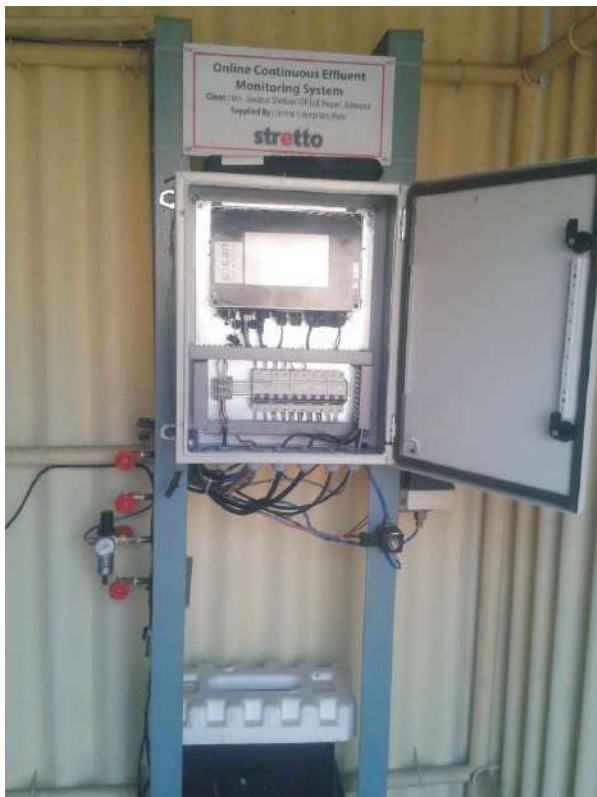
Analyzer for outlet Treated Water - for parameter pH, T.S.S, C.O.D & BOD measurement.
