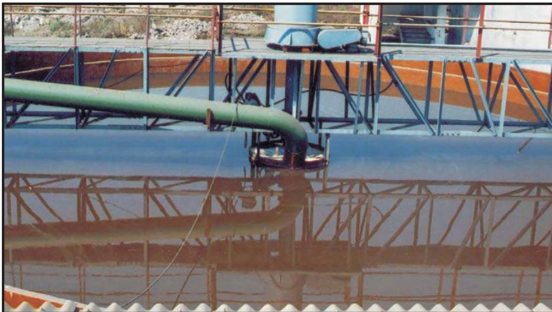
Secondary clarifier new stream
